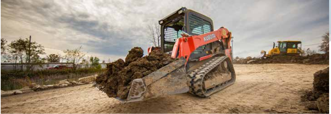
Kubota SVL65-2 operator Rusty Giles came to Performance Training Solutions with limited experience in excavation and running dump trucks. He'll leave the program well positioned for a career in an industry hungry to build on his skill set.
