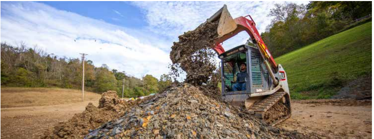
ICR Contracting's Michael Martin moves material—with a Takeuchi TL8 compact track loader—as part of a baseball diamond reconditioning project for Cameron High School, in Cameron, West Virginia. The Dragons hope to be rounding bases on the new field this spring.
