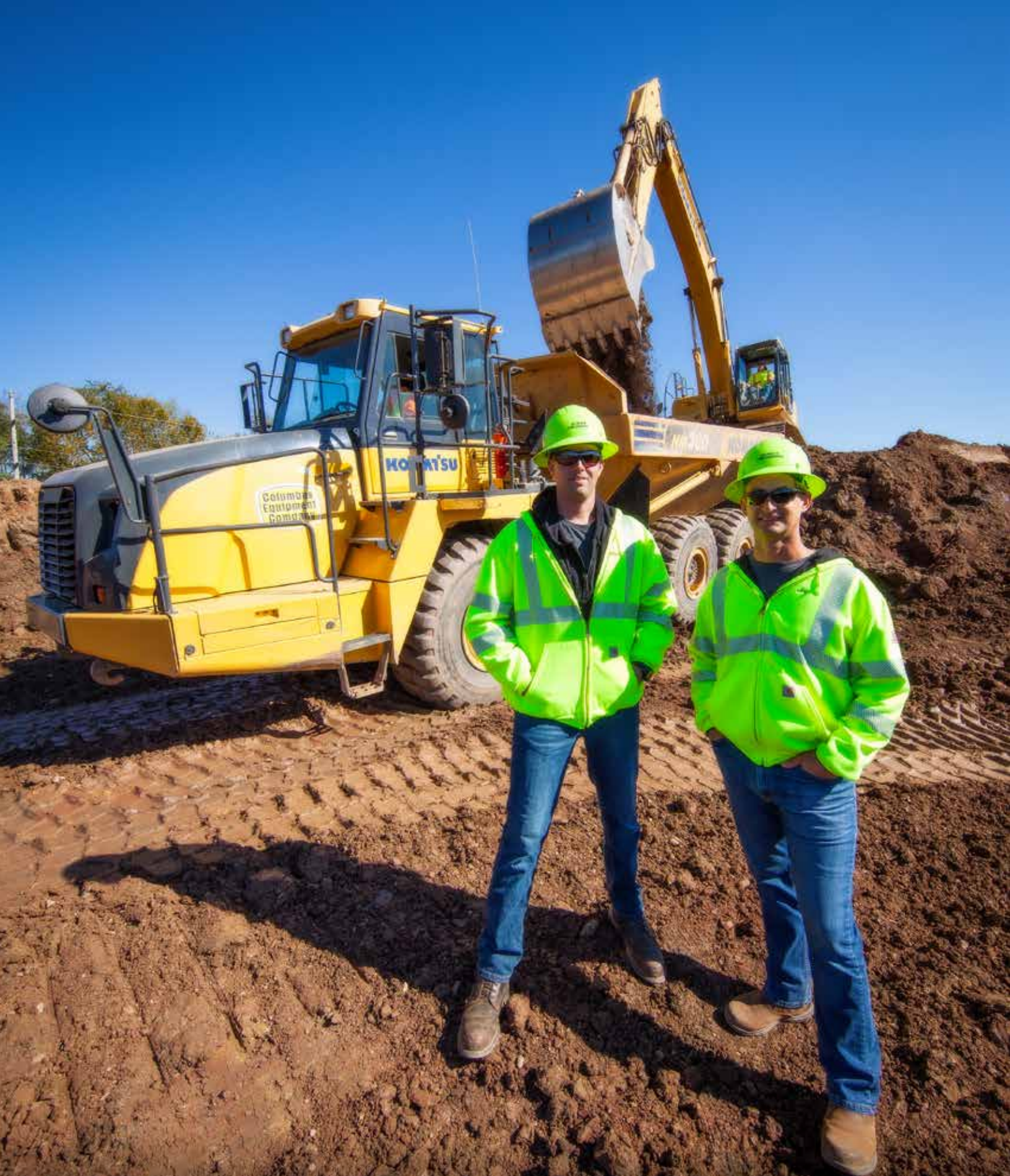
Bedrock Earthworks President Bobby Sykes (left) with Operations Manager Joe Hivnor. Hivnor is a strong proponent of Komatsu technology. "iMC has helped the company grow more and more, control our costs, and eliminate the need for additional employees. Komatsu equipment and Columbus Equipment Company have really inspired this company to grow. We look good in front of our customers, enabling us to secure larger projects and to purchase additional equipment. It's a great win for everybody."
