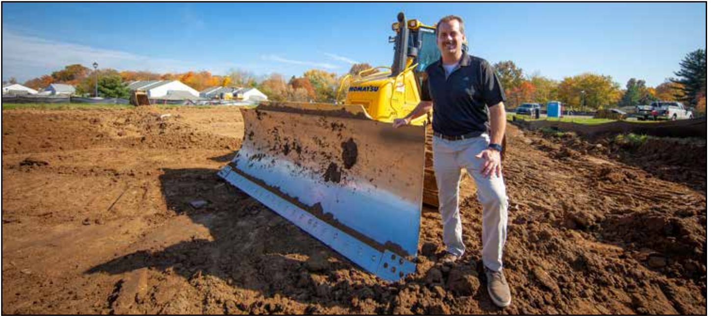
A Crano Excavating President Jim Riter—a third-generation owner—on a residential site development project in Copley, Ohio.
