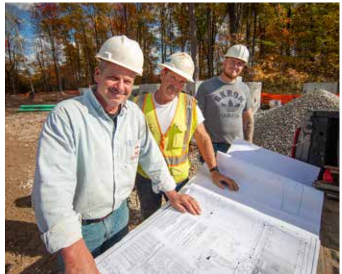
A Crano’s Mike Jones (left) has been with the company 40 years. He leads a crew on a sanitary sewer installation project in Kent, Ohio.
