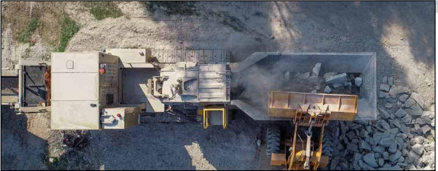
Balsbaugh Excavating's Astec GT440 crushes up to 300 tons of concrete per hour onsite, just outside Englewood, Ohio.
