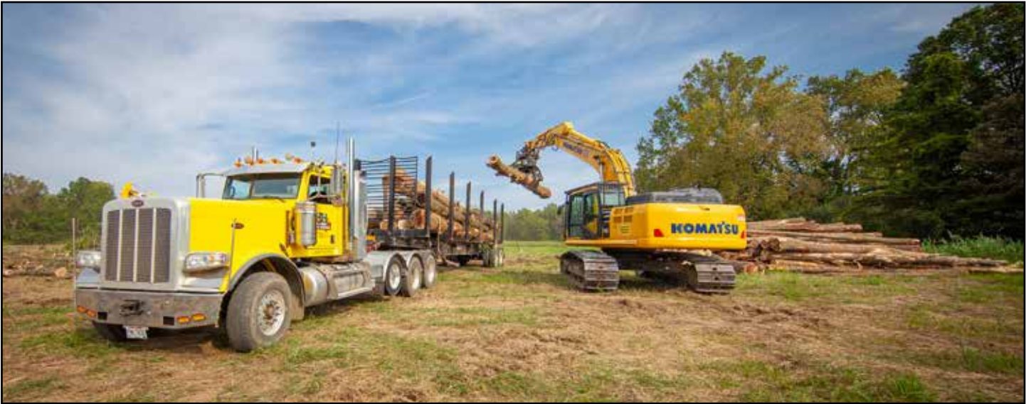
H&H Land Clearing's favorite color: Yellow. A yellow Komatsu PC290LC-11 loads lumber on a residential development site. A CBI 6800CT grinder also just joined the team ... it's yellow too.
