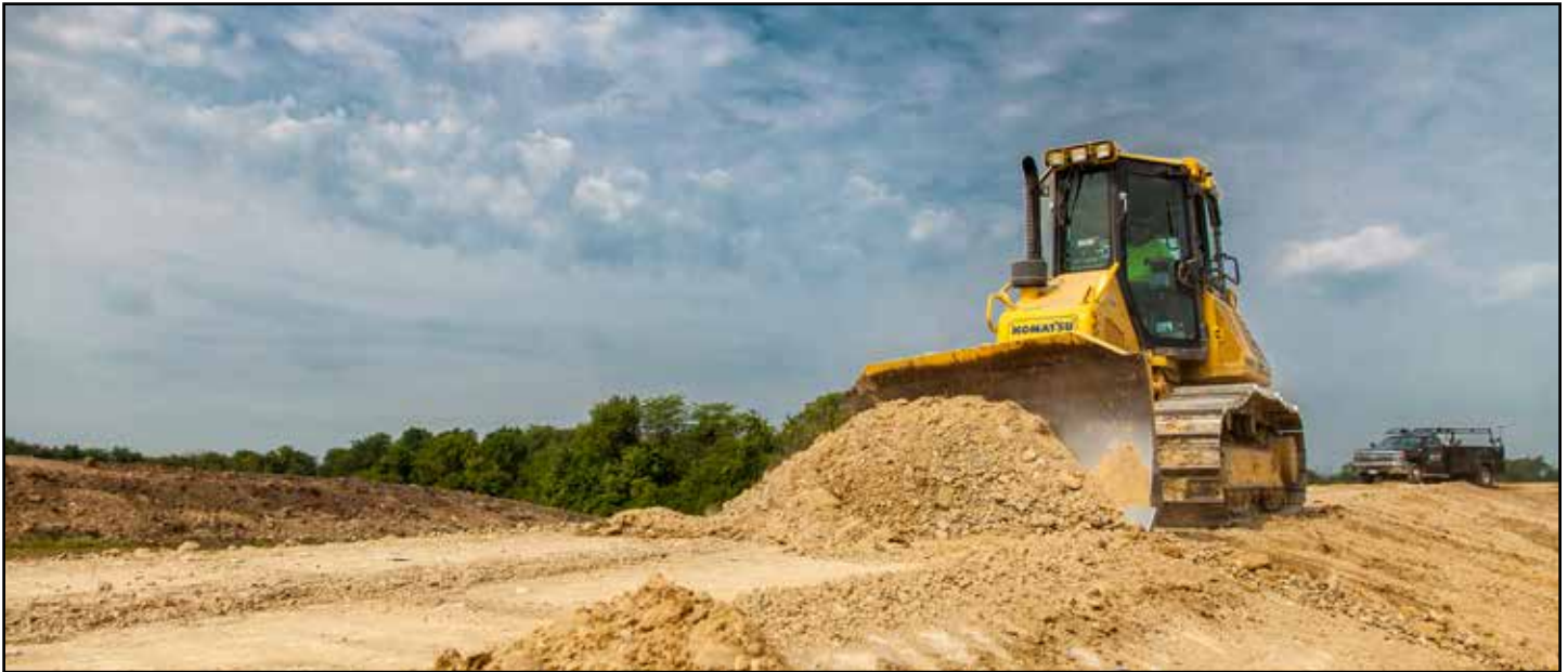
Milcon's Komatsu D51EXi intelligent dozer cutting in a retention pond on the company's $5.4-million Union Village Development Project. Given their experiences with iMC technology—including recently needing 30 trucks to feed the voracious dozers stone on a Dayton International Airport project—Milcon crews have rightly come to depend upon “phenomenal production” from the equipment.
