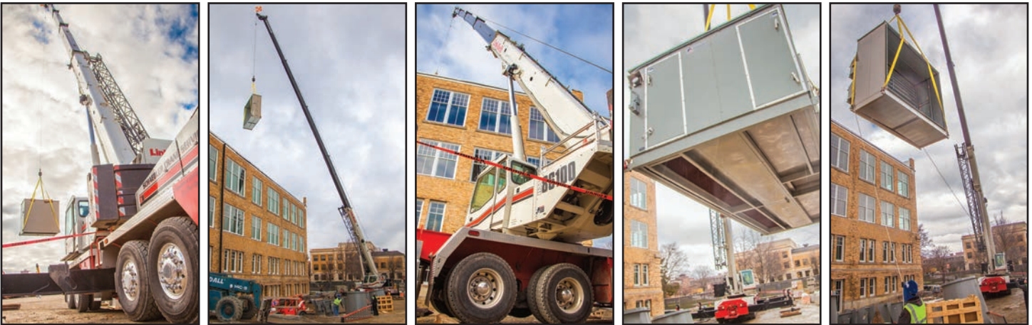
Installation of the 30,000-lb., air-handling system at the science facility required two days and approx. 20 lifts. The six-stage process involves lifting an 8,500-lb. supply air fan, a spacer, coil section, filter system, economizer and pipe portal to the building's roof for assembly.
