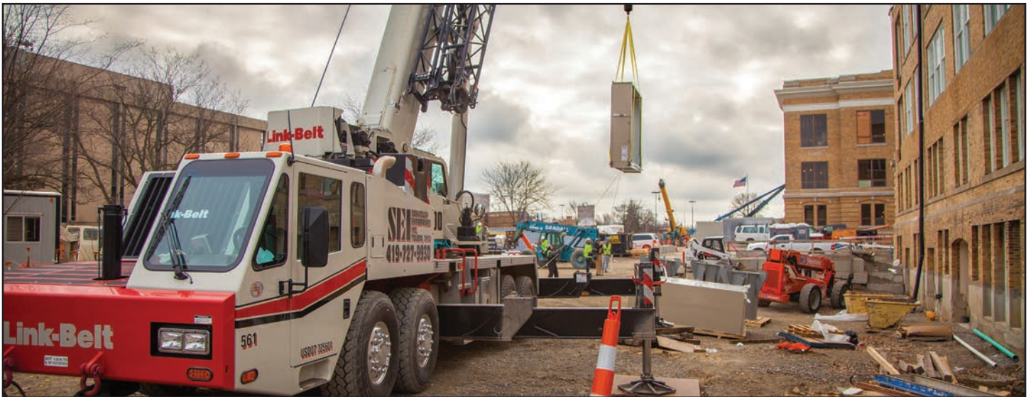
SEI Schaedler's Link-Belt HTC-86100 Operator Art Cole and crew lift one component of a Daikin Supply Air System as part of the $23-million renovation of BGSU's Moseley Hall in Bowling Green, Ohio. The project is scheduled for completion by June 2017.
